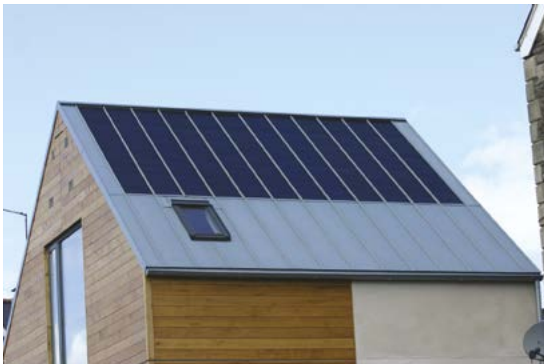
21 | Solar panels, Coach House, Cardiff
