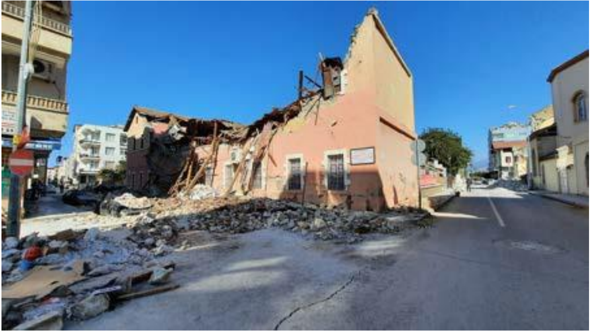
The former French Embassy, which is used as Iskenderun Mithatpaşa Secondary School, was damaged after the earthquake.
