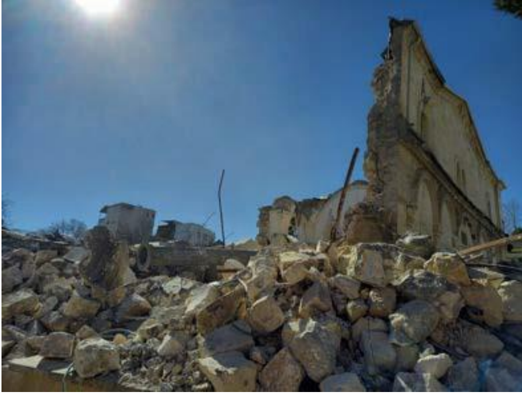
Damages observed in Adiyaman Ulu Mosque after the earthquake (Photograph: Assoc. Prof. Dr. Koray Güler)
