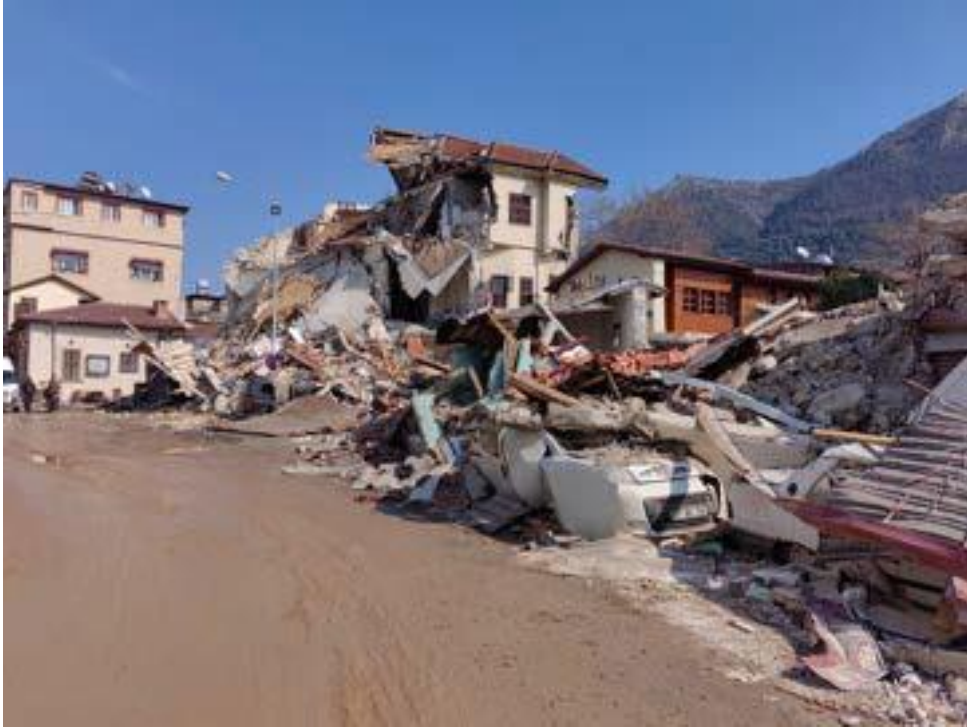
Examples of damages to civil architecture works in the historical city centre of Antakya after the earthquake of 20 February 2023 (Photograph: Assoc. Prof. Dr. Koray Güler)
