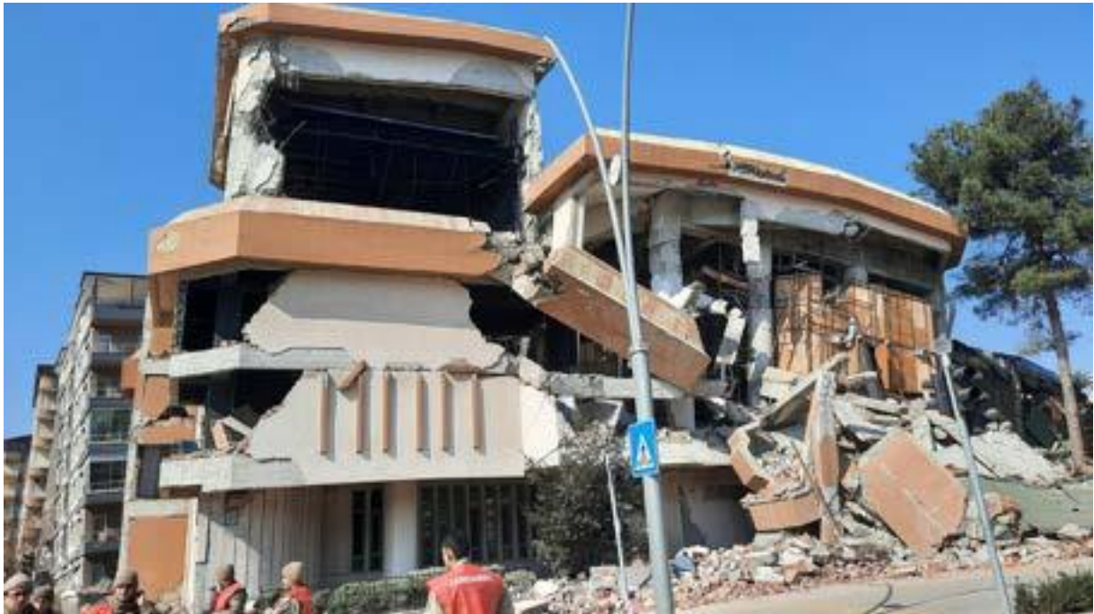
Damage to Hatay Cultural Centre after the earthquakes of 6 February 2023
