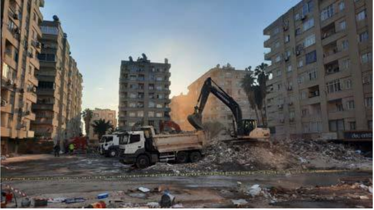
Osmaniye - Metin Tamer Site after earthquake
