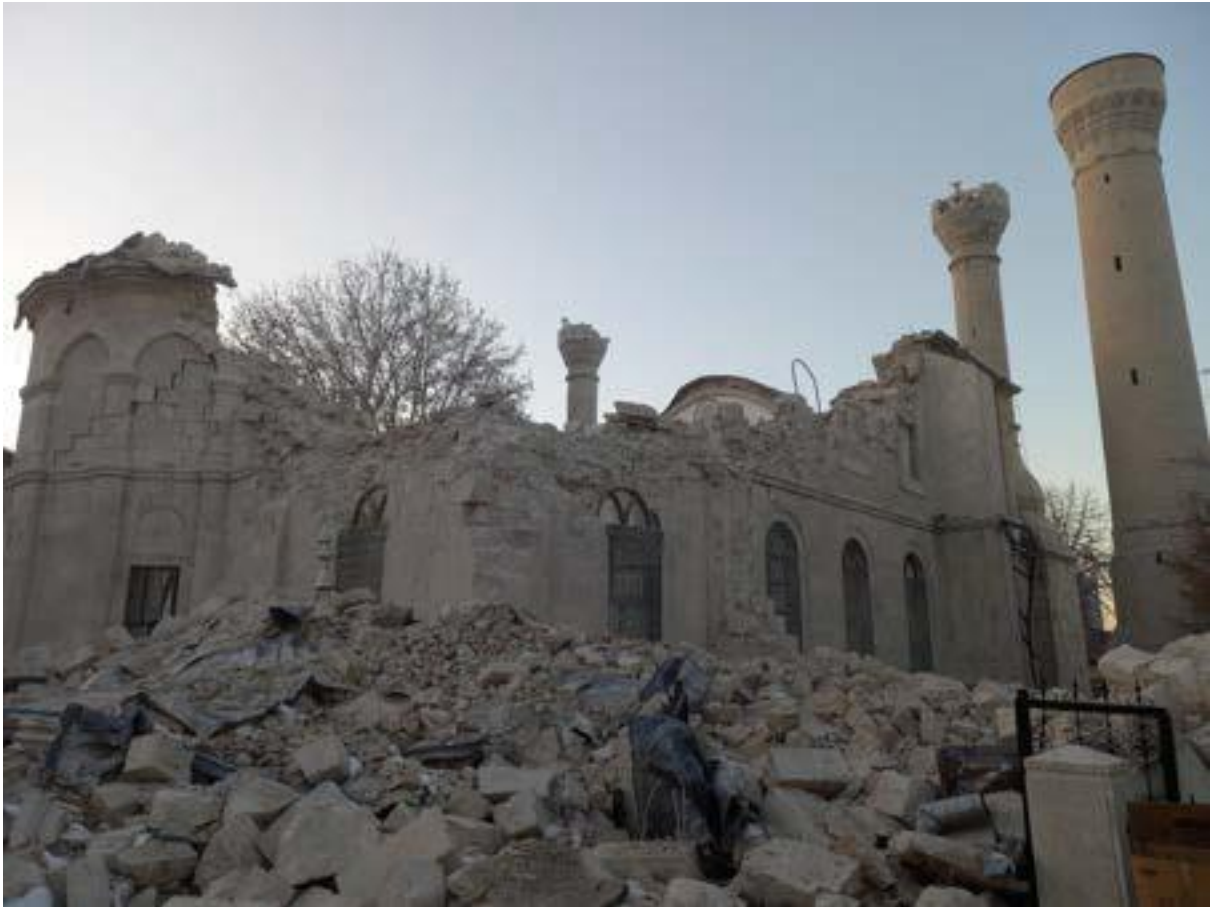
Damages observed in Malatya Ulu Mosque after the earthquake (Photograph: Assoc. Prof. Dr. Koray Güler)
