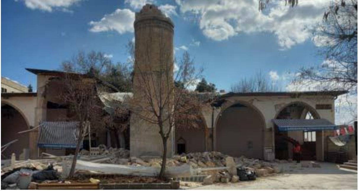
Damages observed in Kahramanmaraş Ulu Mosque after the earthquake (Photograph: Assoc. Prof. Dr. Koray Güler)
