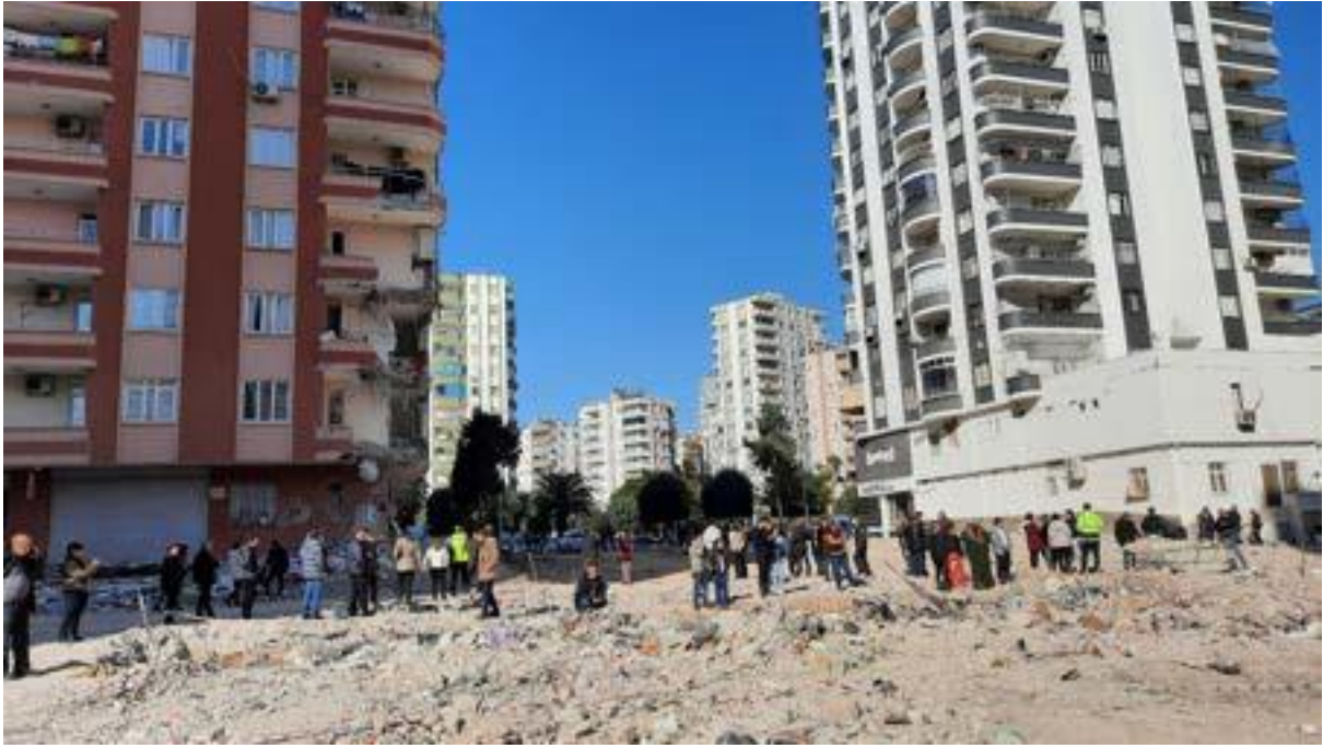
Adana - City centre demolished buildings
