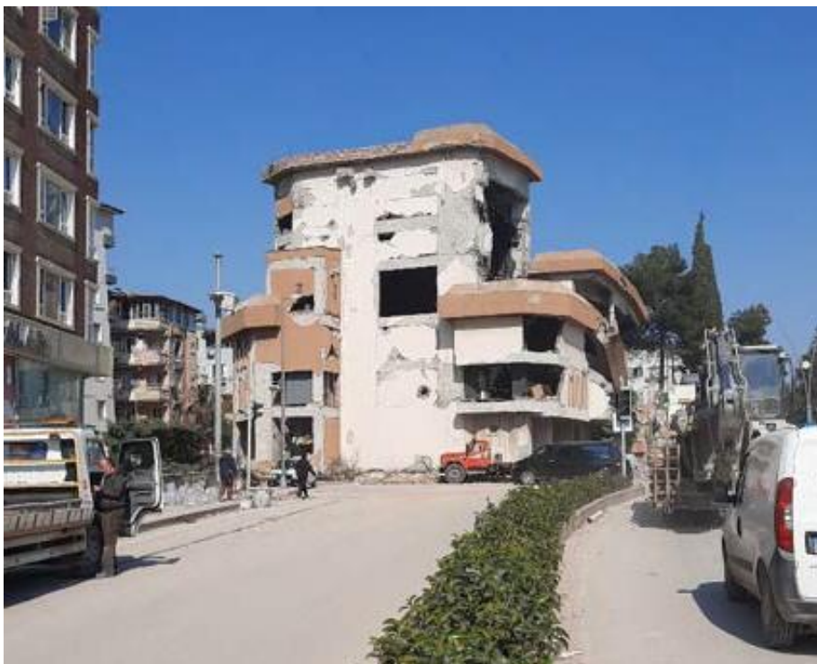
Damage to Hatay Cultural Centre after the earthquakes of 6 February 2023
