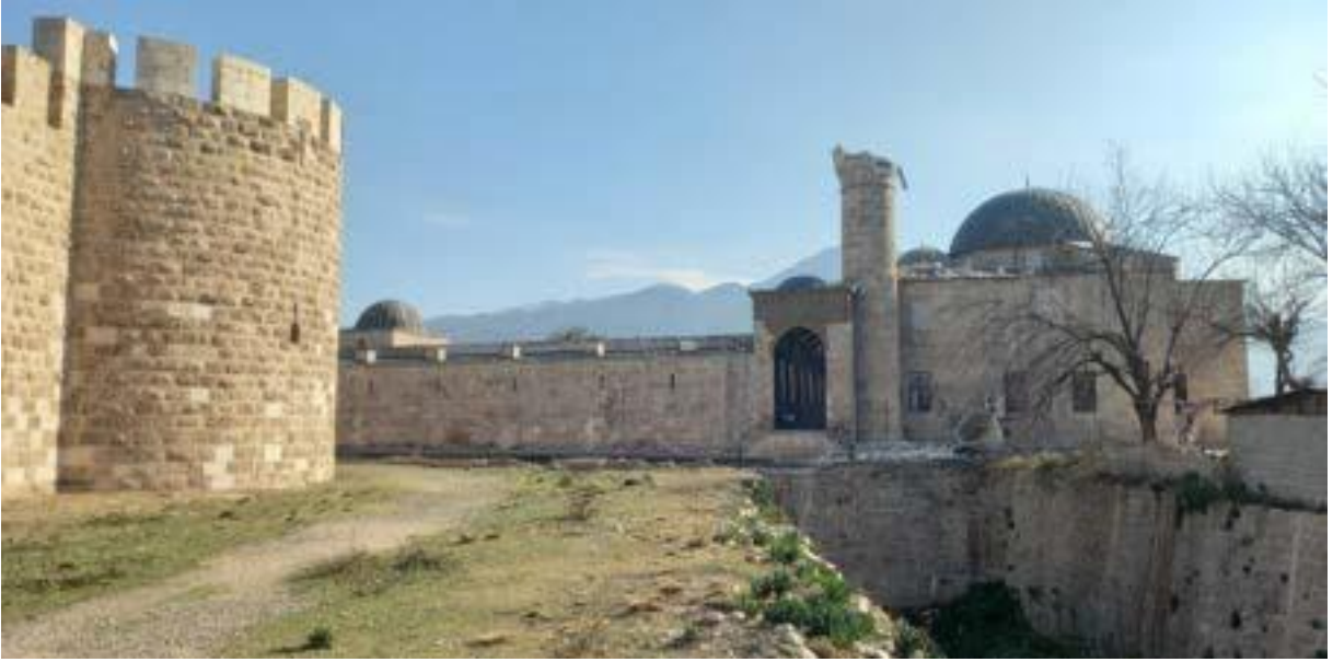
Damages observed in Payas Sokollu Mosque after the earthquake (Photograph: Assoc. Prof. Dr. Koray Güler)
