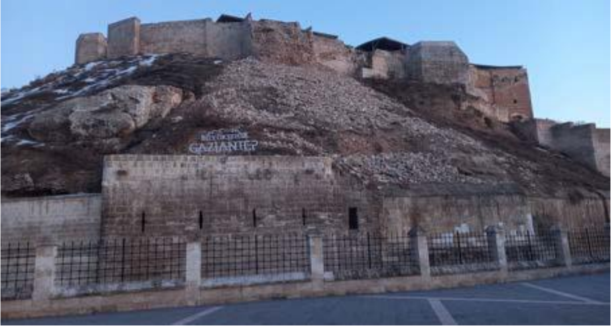
Damages observed in Gaziantep Castle after the earthquake (Photograph: Assoc. Prof. Dr. Koray Güler)
