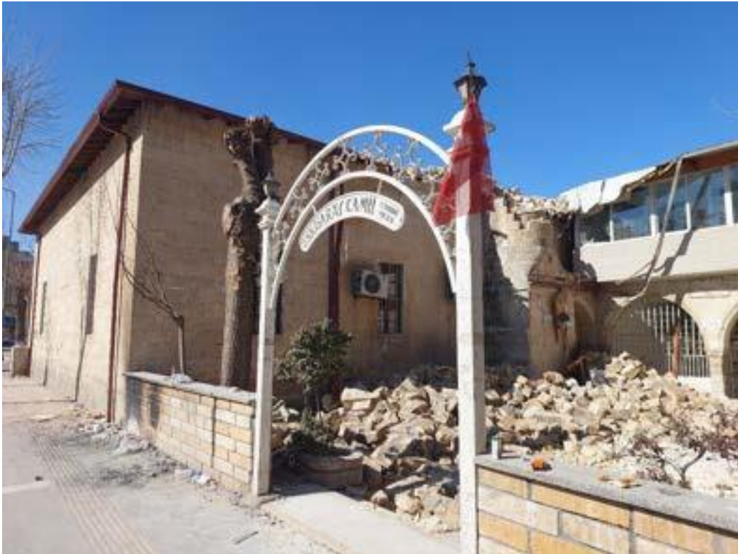
Damages observed in Adiyaman Eski Saray Mosque after the earthquake
