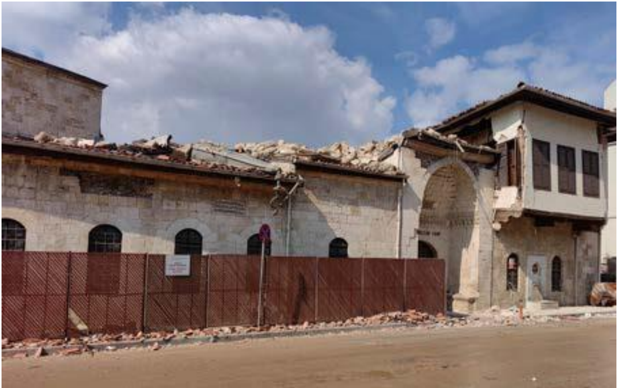
View of Habib-i Neccar Mosque, Hatay, after the earthquake of 20 February 2023
