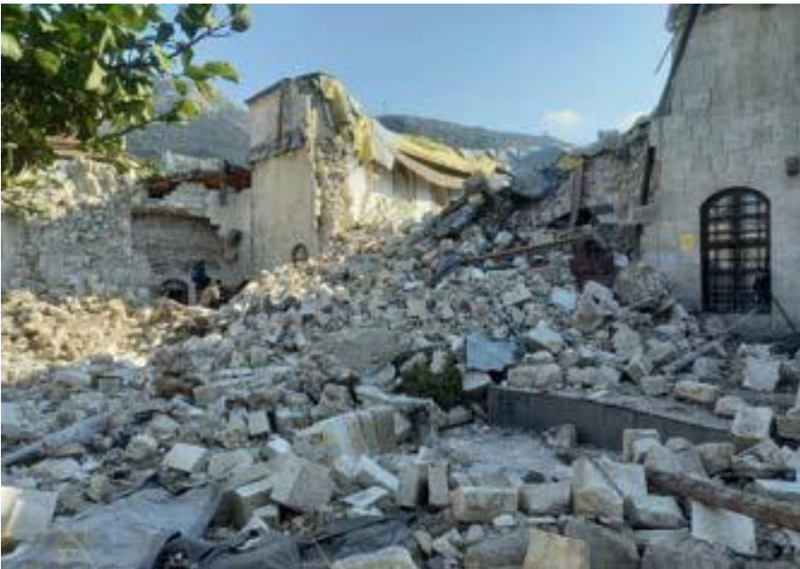
The view of Habib-i Neccar Mosque in Hatay after the earthquakes of 6 February 2023
